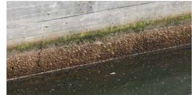
Heavy leaching and damage to the structural concrete are observed particularly in the water splash zone of biological treatment basins.
