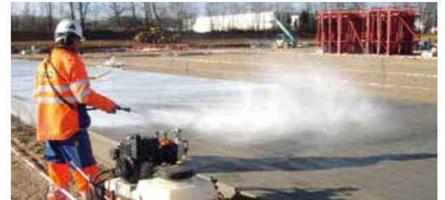
Immediate coverage or curing of concrete surfaces exposed to the elements is the most crucial step for protection of such surfaces.
