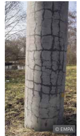
The appearance of ASR damage can be assessed very well on the drying concrete surface of this bridge pylon. Damage can appear within years or only after decades.
