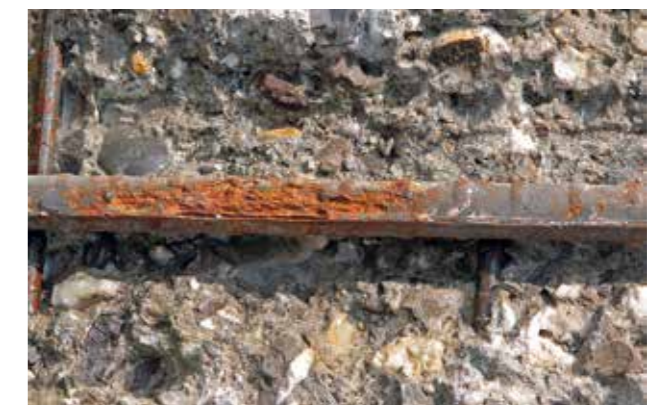
Damage to concrete structure due to insufficient concrete cover and low concrete quality
