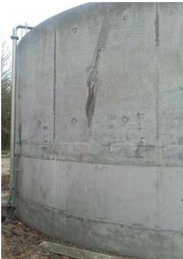
Crack bridging before reinforcement
