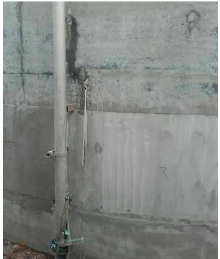
Fluid leaks before and during repair.
